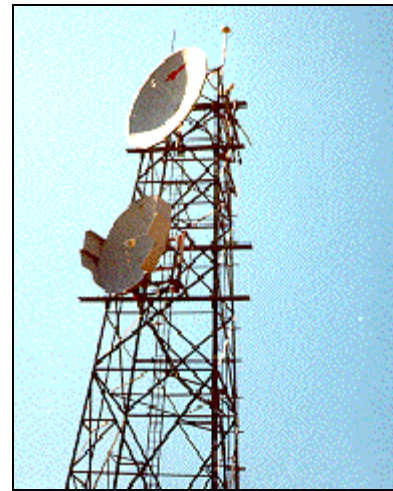
Figure 5. Photograph of IGS Goldstone Antenna Installation. According to the site log, the GPS antenna is mounted on top of a 25 meter, unguided Microwave tower, within 100 meters of the MARS 70 meter diameter Deep Space Antenna [23].
